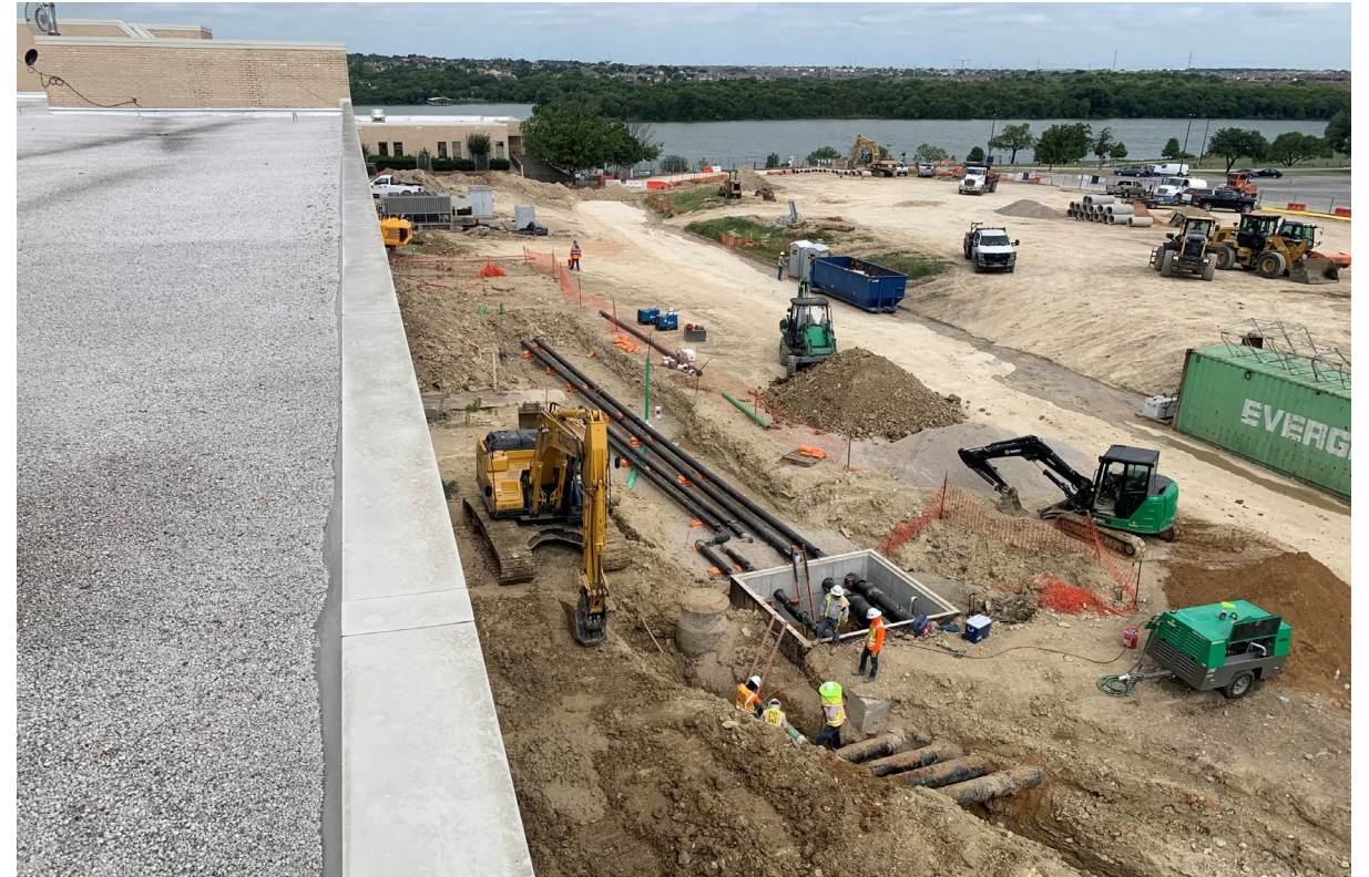
GMP 1: Summit Vault with thermal 4-pipe system completed! Back filling for concrete pour throughout corridor.
