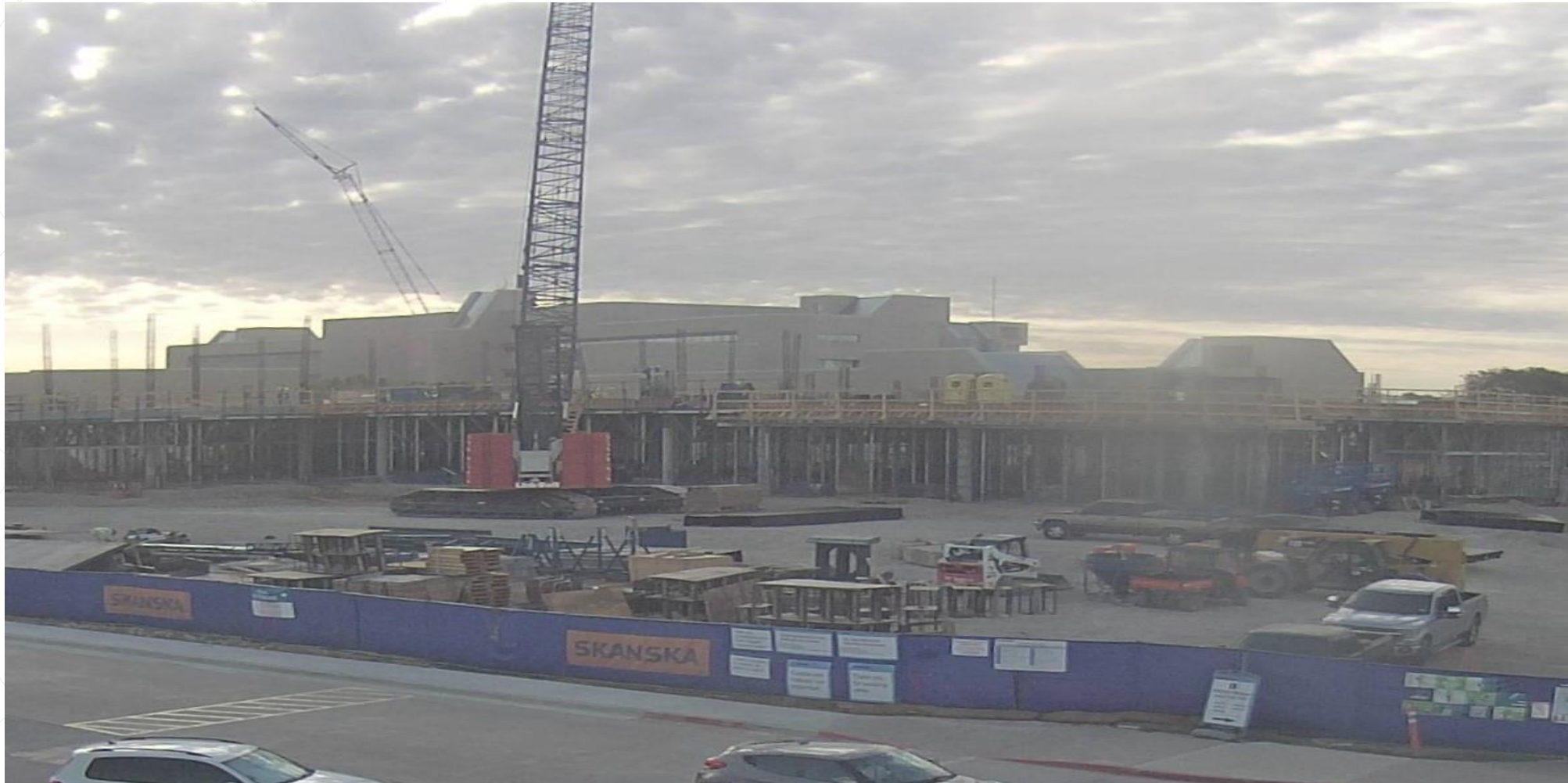
GMP-3: (Looking Northwest) Building 1 second floor slab concrete placement ongoing; third floor concrete column rebar cages
