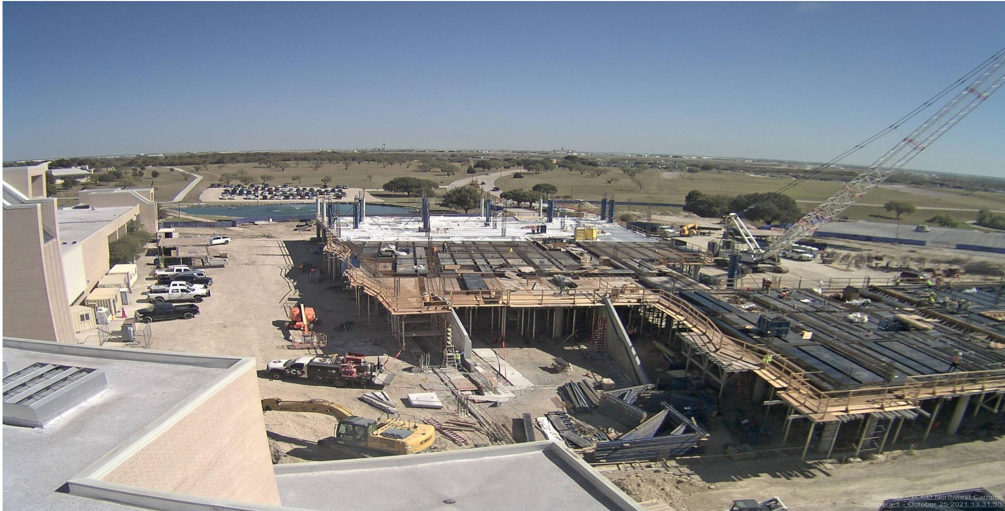
GMP-3: (Looking East) Building 2 second floor slab rebar installation; rebar cages for concrete column supports for third floor slab starting
